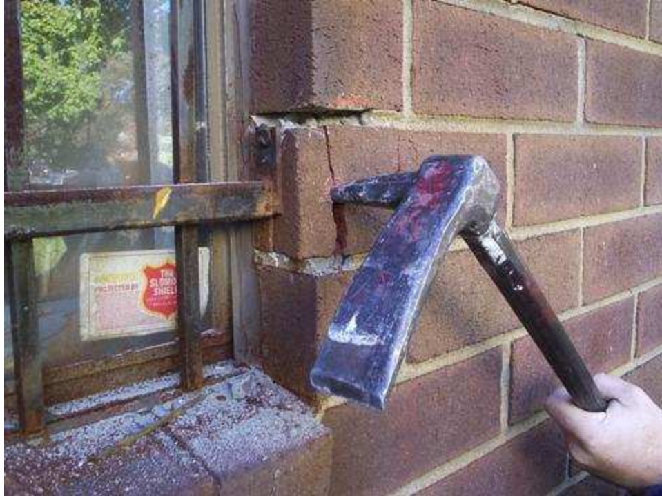
Our initial inspection shows us that we have security bars that are secured into a brick wall on the inside of the window opening. One well placed strike from irons (using pike of the halligan), quickly shows us what we want to find... "the weakest link."
