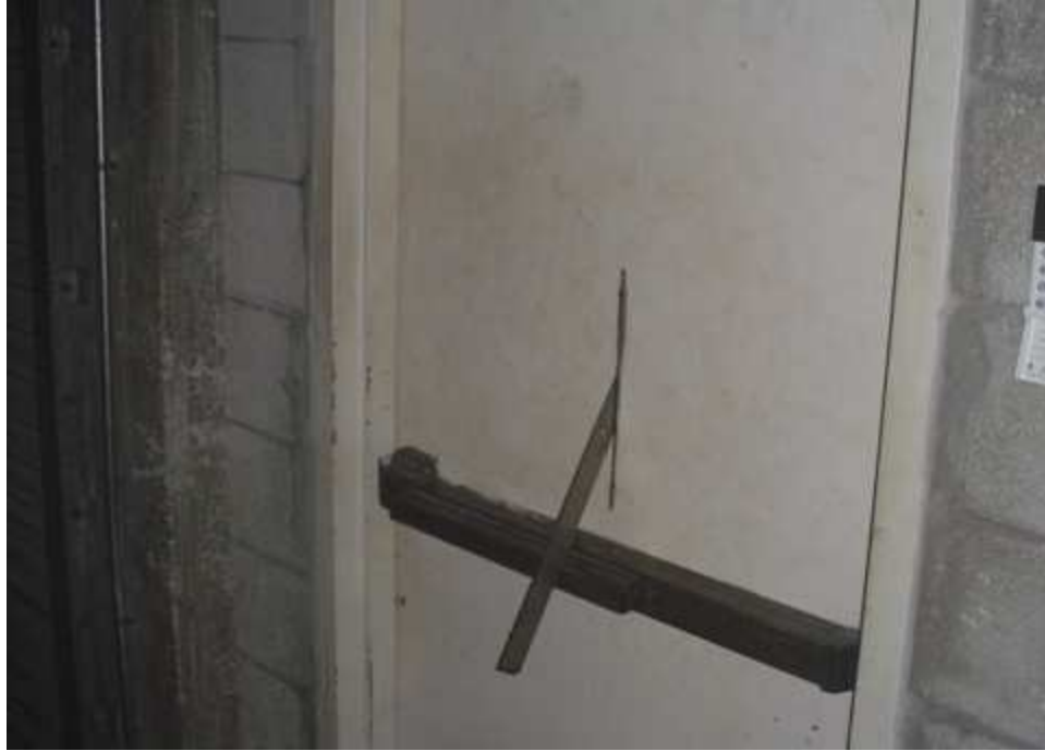
A view from the inside shows how the framing square is utilized to manipulate the panic hardware.
