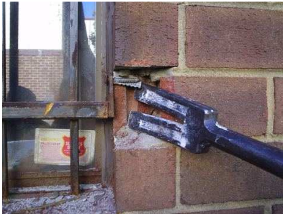
After a few strikes of the irons, the entire anchor will be exposed. The exposed anchor can then be pried out with the fork of the halligan.
